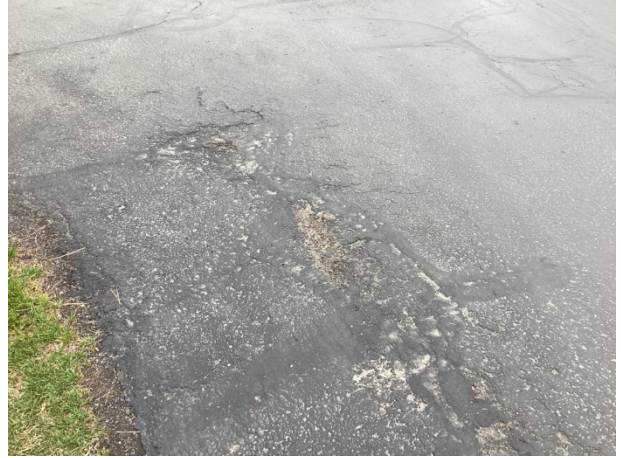
Pavement cracks at Smoochers Circle
