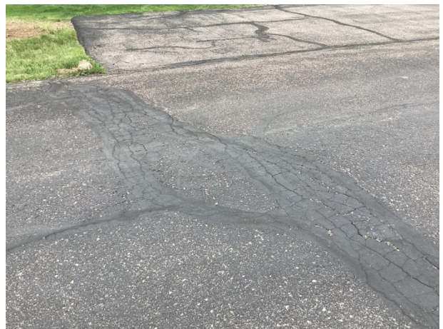
Pavement cracks at Hillbrook Lane
