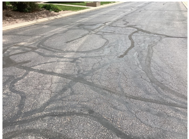
Pavement cracks at Camel Grove
