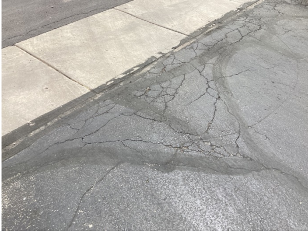
Pavement cracks at Sheiks Place
