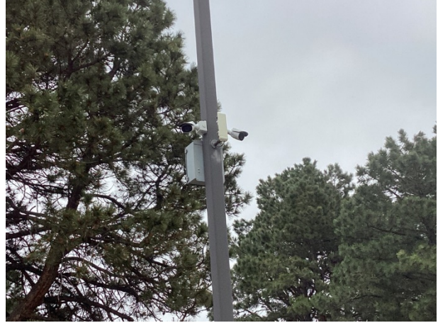
Security system cameras
