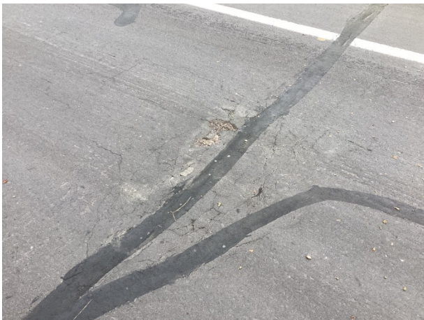
Pavement cracks at Kissing Camels Drive
