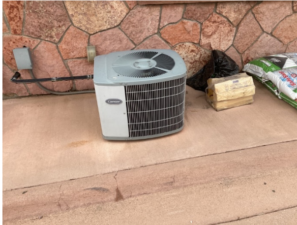
Guard house condensing unit
