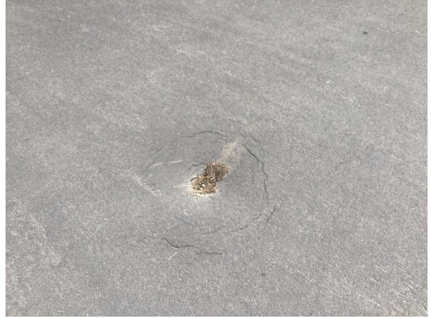
Pavement cracks and settlement at Kissing Camels Drive
