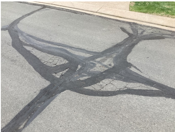
Pavement cracks at Camelrock View
