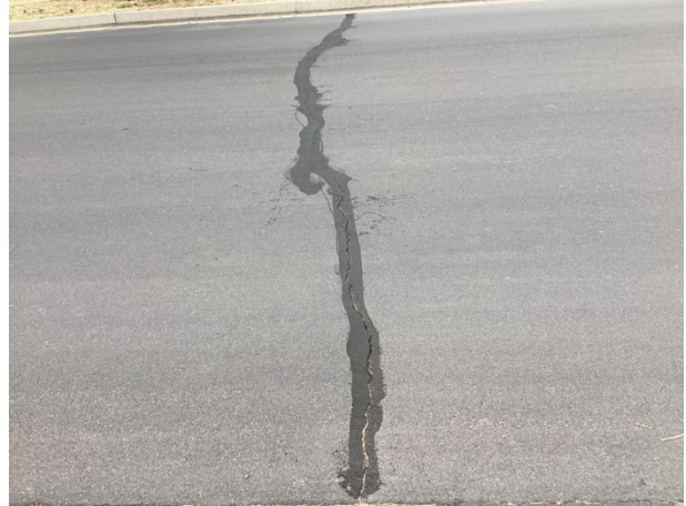
Pavement cracks at Hill Circle
