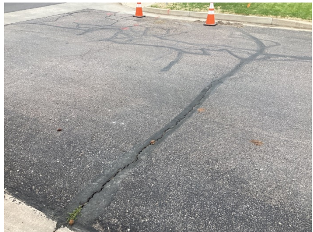
Pavement cracks at Cumulus View
