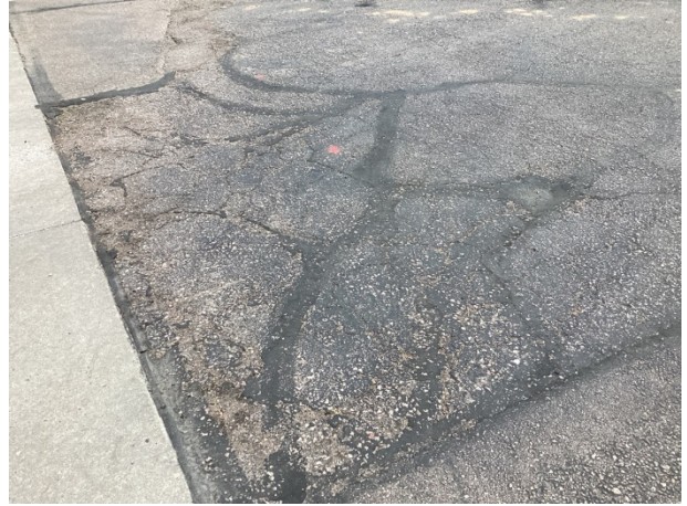
Pavement cracks at Edge Cliff Court
