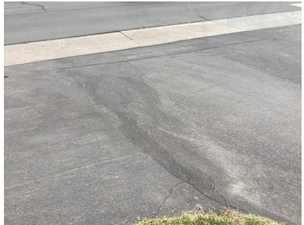
Pavement cracks at Kissing Camels Drive
