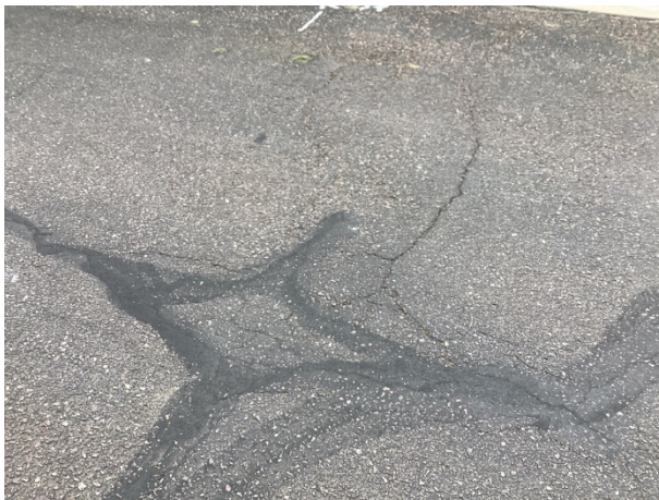
Pavement cracks at Moonrise Court
