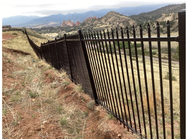
Fence leaning section
