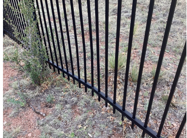
Fence picket damage
