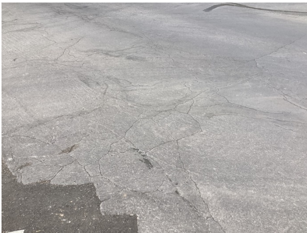
Pavement cracks at Kissing Camels Drive
