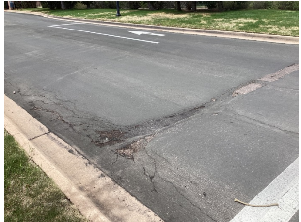
Pavement cracks at the west residential entrance
