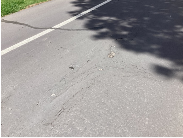
Pavement cracks at Kissing Camels Drive
