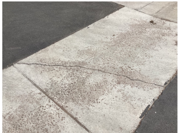
Concrete cracks at Hill Circle
