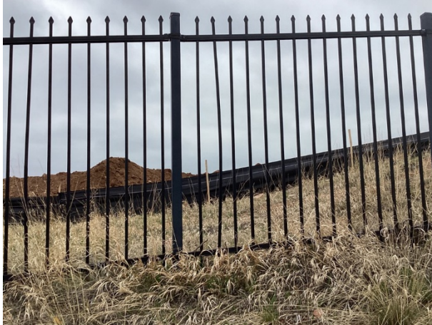
Fence picket damage
