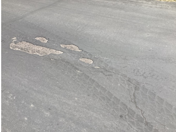
Pavement cracks and deterioration at Kissing Camels Drive
