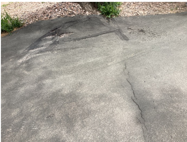
Pavement cracks at Sunnybrook Lane
