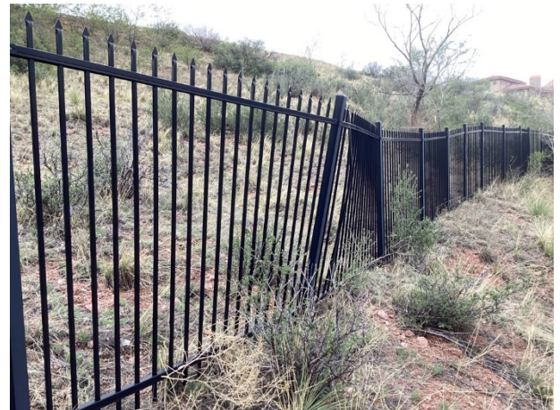
Fence leaning section
