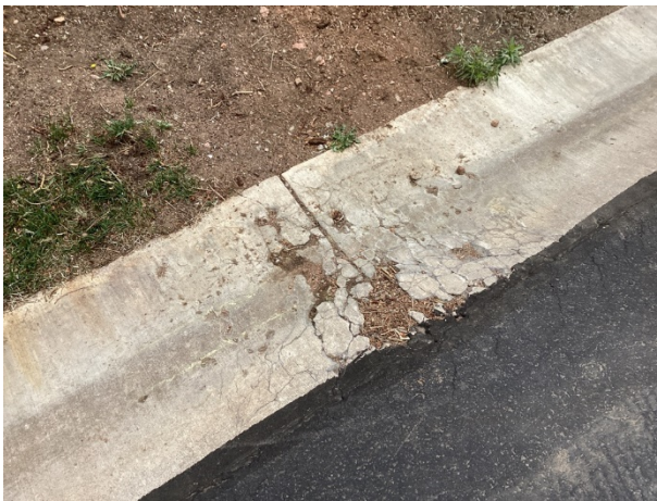
Concrete cracks and damage at Smoochers Circle
