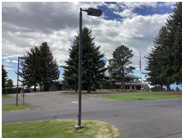
Light pole and fixture
