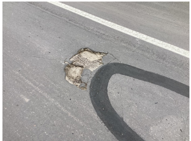
Pavement cracks and pot hole formation at Kissing Camels Drive
