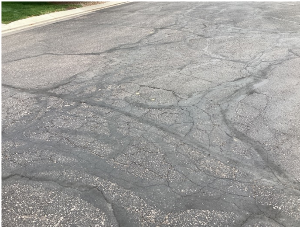
Pavement cracks at Alta Mesa Court
