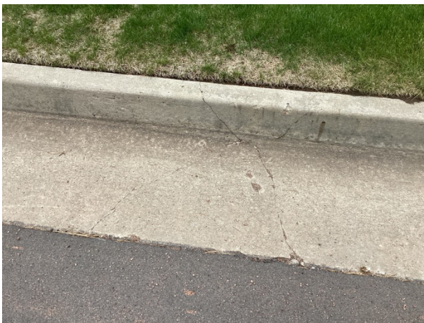
Concrete cracks at Hill Circle
