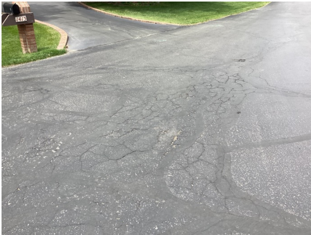
Pavement cracks at Smoochers Circle
