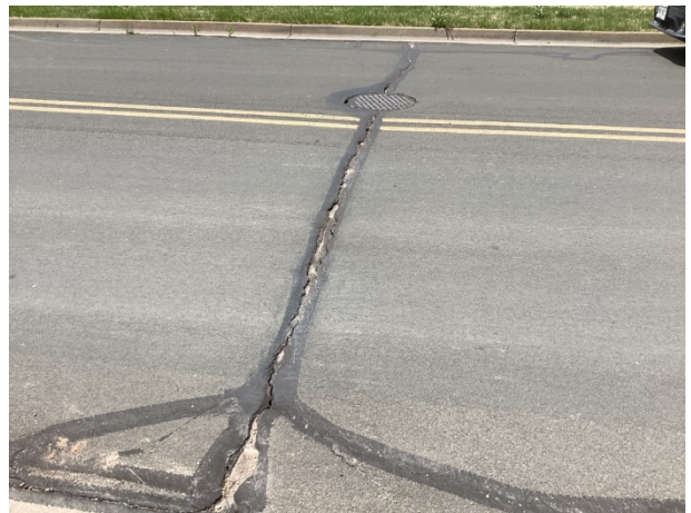
Pavement cracks at the east entrance street
