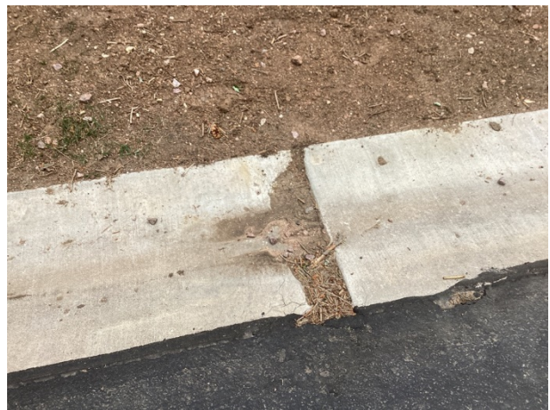
Concrete damage at Smoochers Circle
